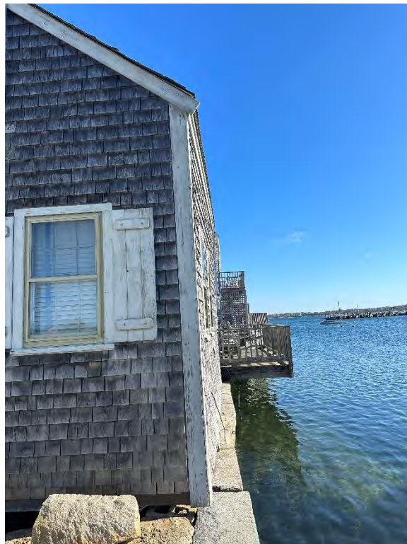
Photo 8 - Waterside bearing wall bow
