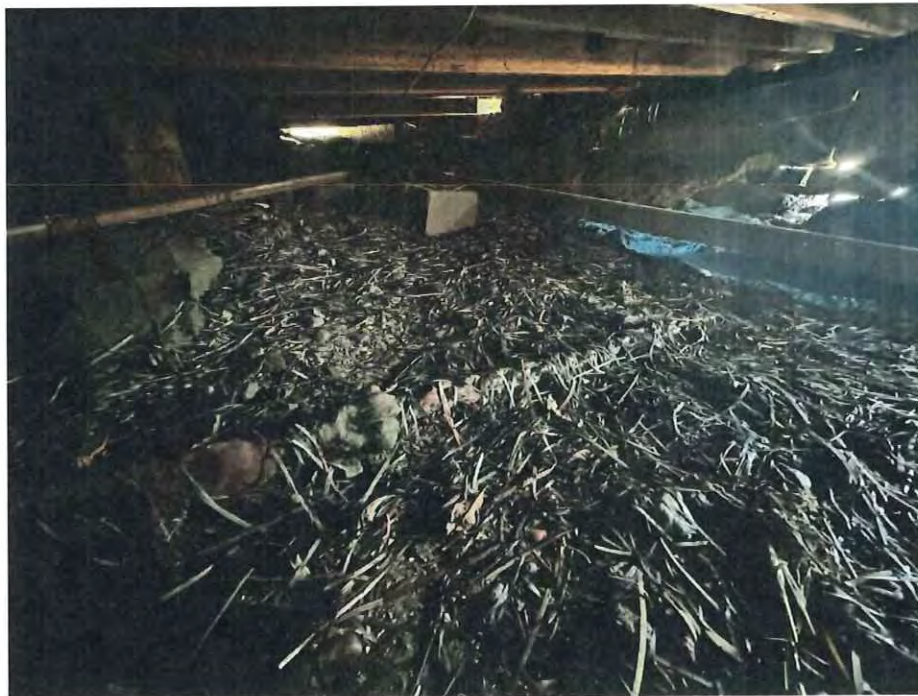
Photo 23 - Evidence of constant water intrusion (Crawl Space)
