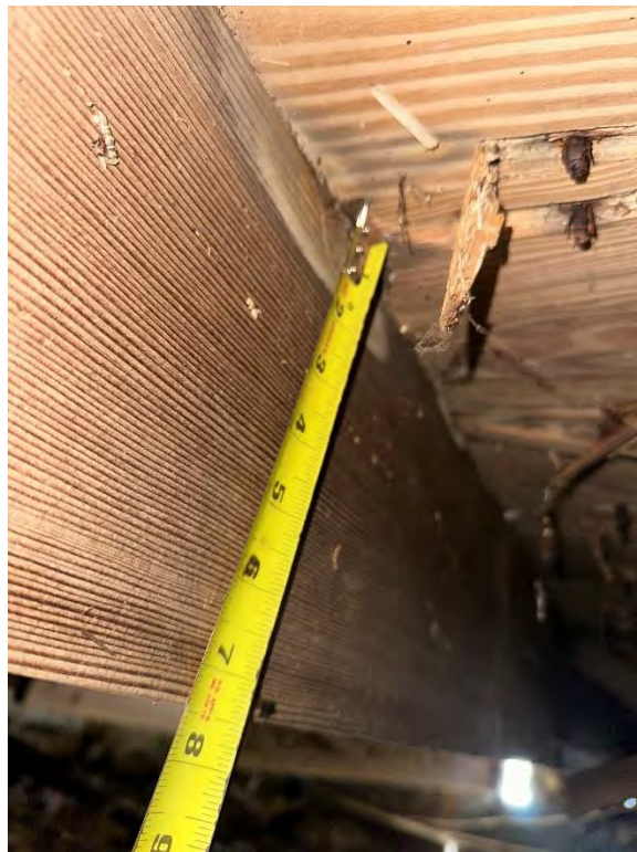
Photo 33 - 2x8 floor joists @ 16" o.c. undersized (Crawl Space)
