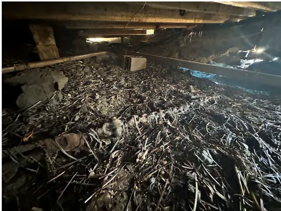
Photo 23 - Evidence of constant water intrusion (Crawl Space)
