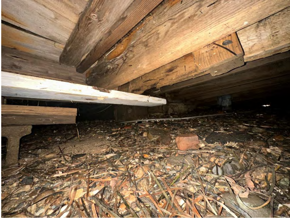
Photo 24 - Floor joist failure and fixes (Crawl Space)
