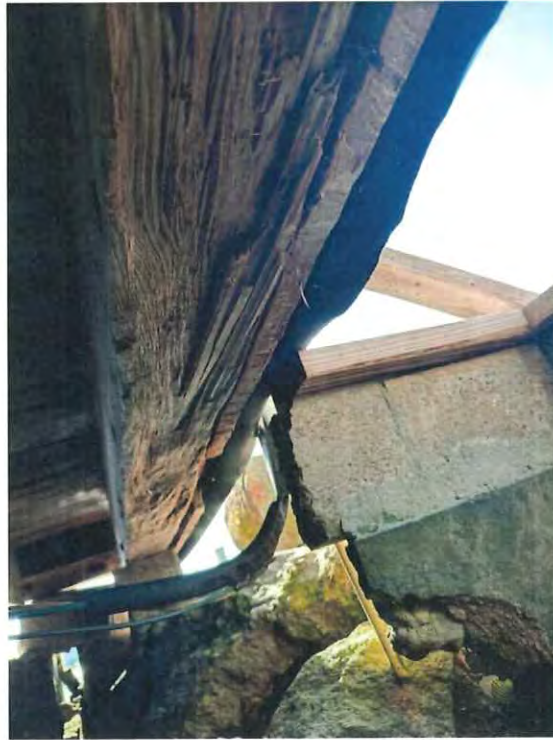
Photo 32 - Support end sill beam rot (Crawl Space)
