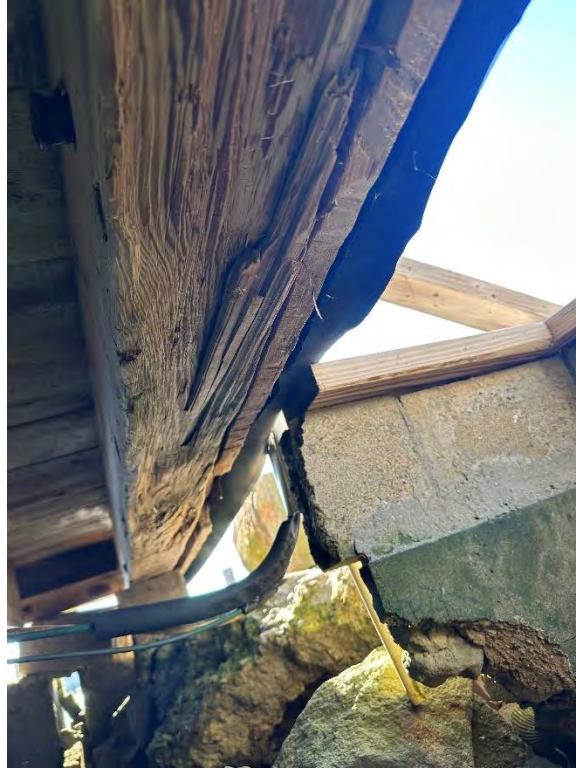
Photo 32 - Support end sill beam rot (Crawl Space)
