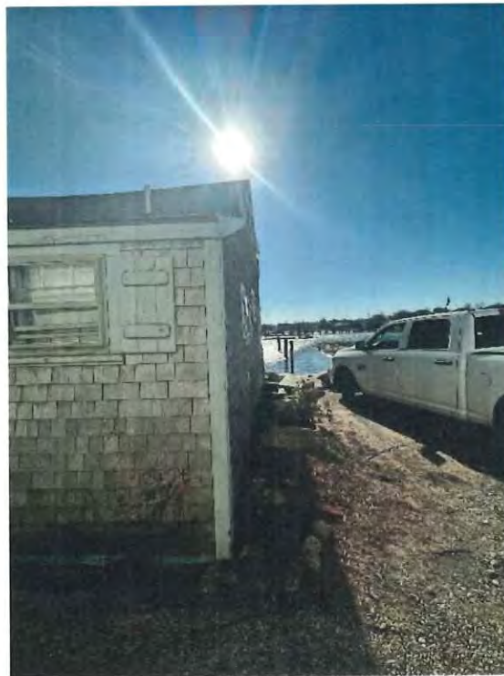
Photo 10 - Petral landing gable end wall bow
