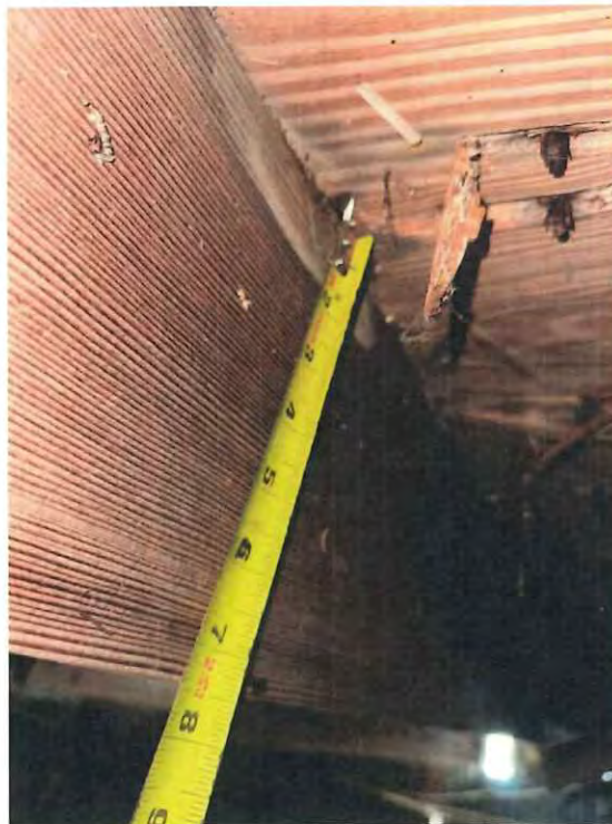
Photo 33 - 2x8 floor joists @ 16" o.c. undersized (Crawl Space)
