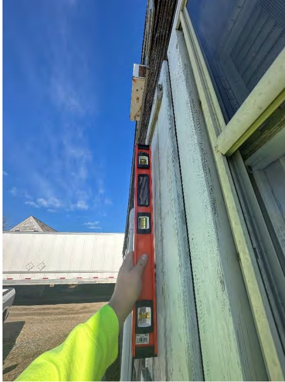
Photo 11 - Petral landing gable end wall bow
