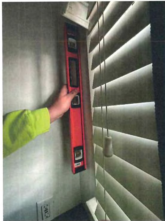
Photo 17 - Gable wall bow Kitchen (Interior)
