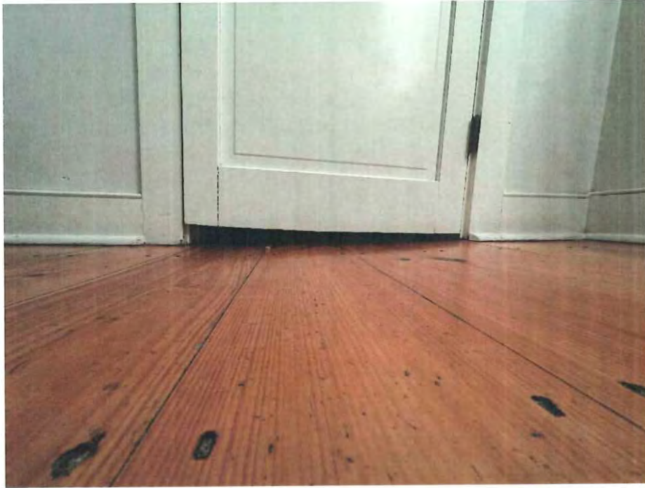
Photo 15 - Waterside bedroom floor slope (Interior)
