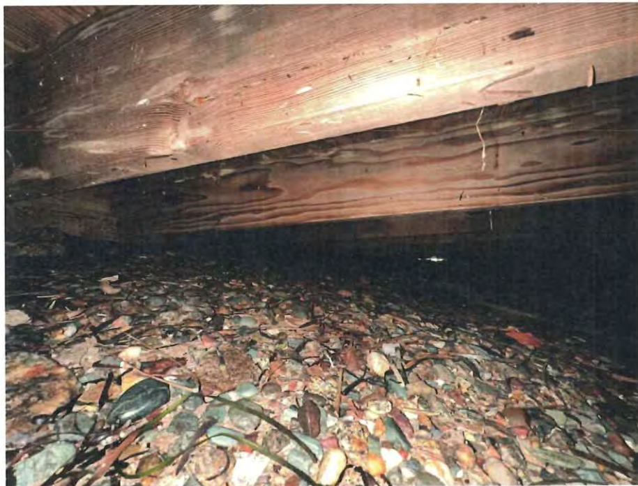
Photo 25 - Exterior support beam buried under sand/dirt (Crawl Space)
