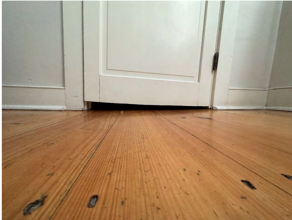
Photo 15 - Waterside bedroom floor slope (Interior)
