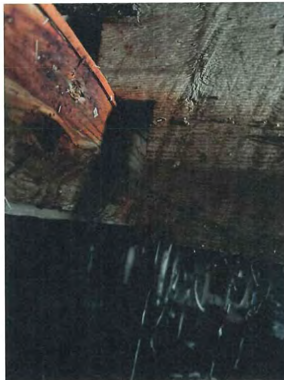
Photo 27 - Notched joists falling off support end sill beam (Crawl Space)
