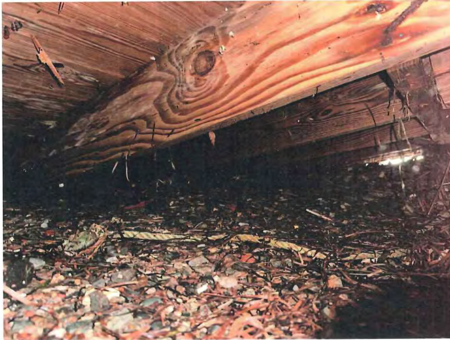
Photo 26 - Floor joists/support beam buried under sand/dirt (Crawl Space)
