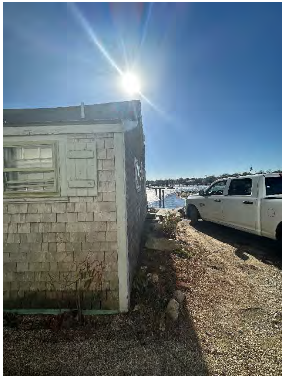
Photo 10 - Petral landing gable end wall bow
