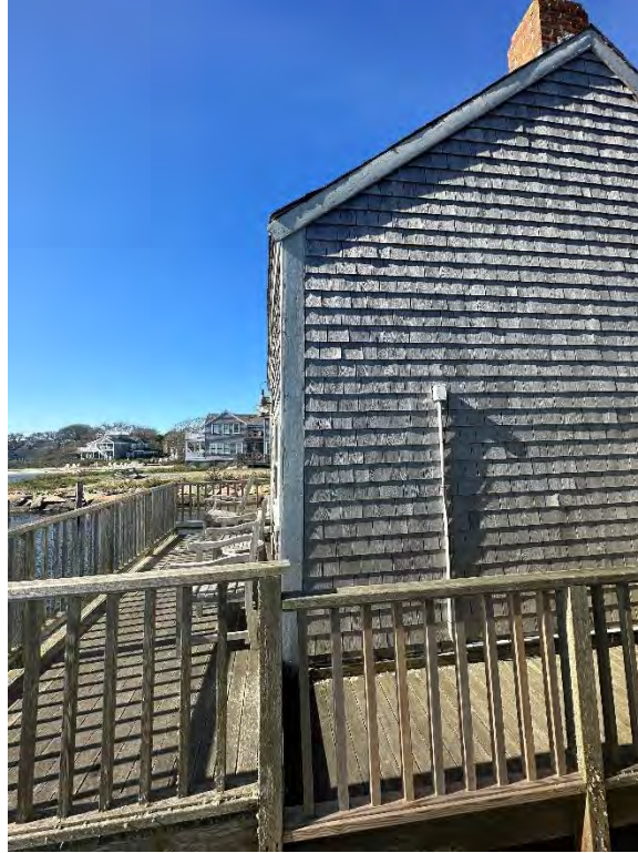
Photo 9 - Waterside bearing wall bow
