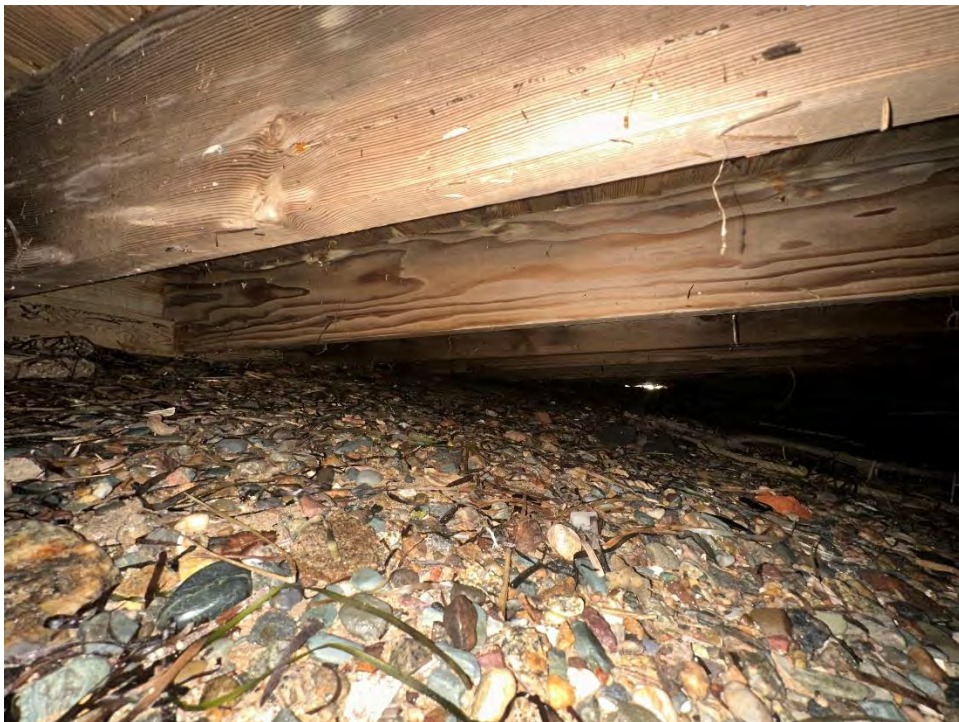
Photo 25 - Exterior support beam buried under sand/dirt (Crawl Space)
