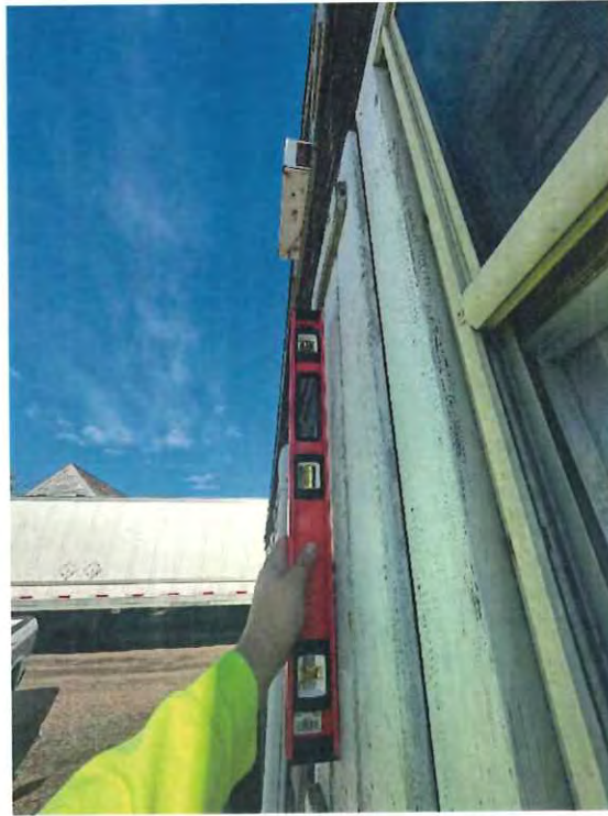
Photo 11 - Petral landing gable end wall bow
