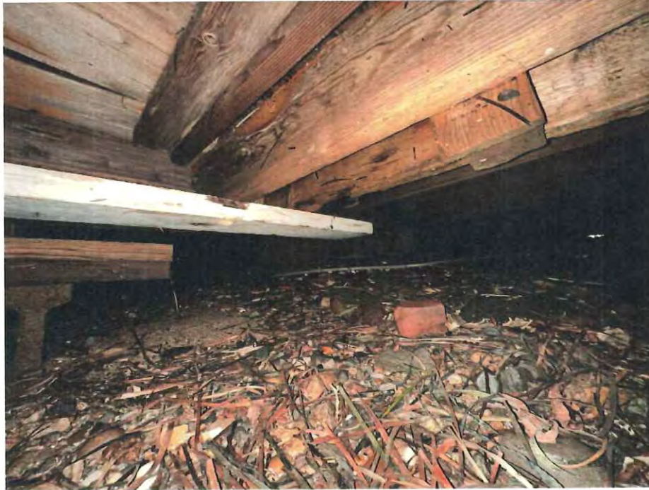
Photo 24 - Floor joist failure and fixes (Crawl Space)
