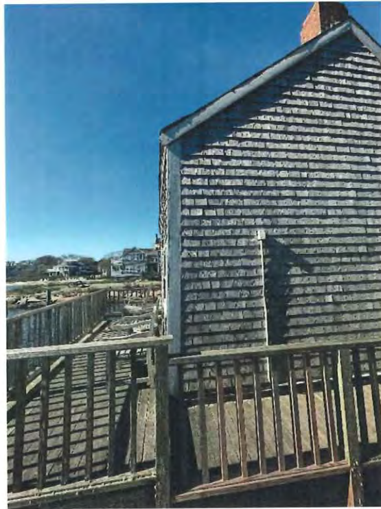
Photo 9 - Waterside bearing wall bow
