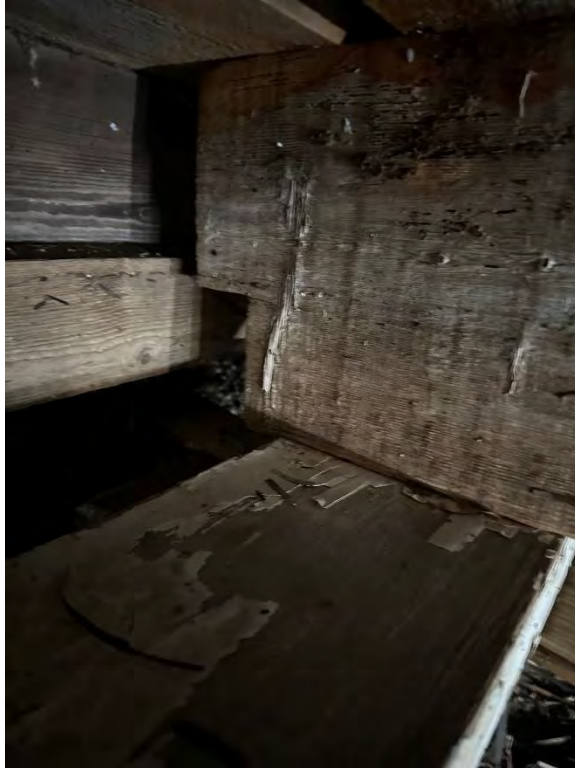
Photo 30 - Notched joists off support end sill beam (Crawl Space)
