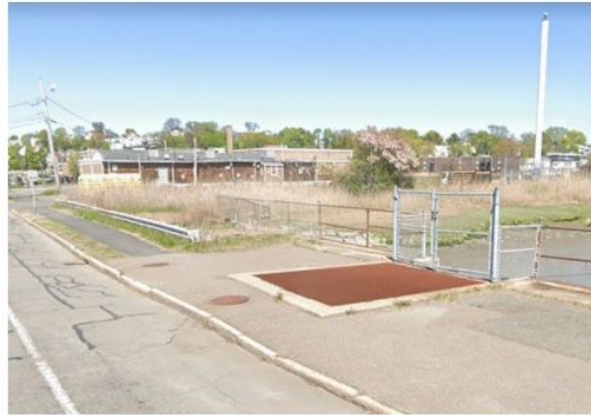
Belle Isle Inlet tide gate at the border between Boston and Revere (looking northeast)
