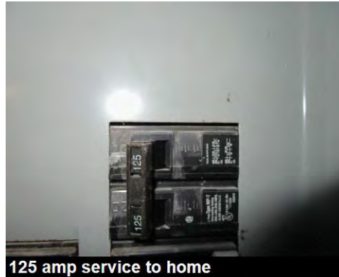
125 amp service to home
