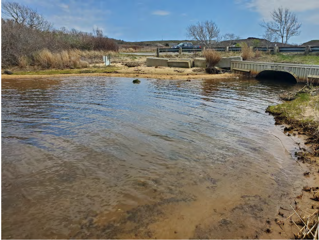
Figure 5. Overview with unstable bank.
