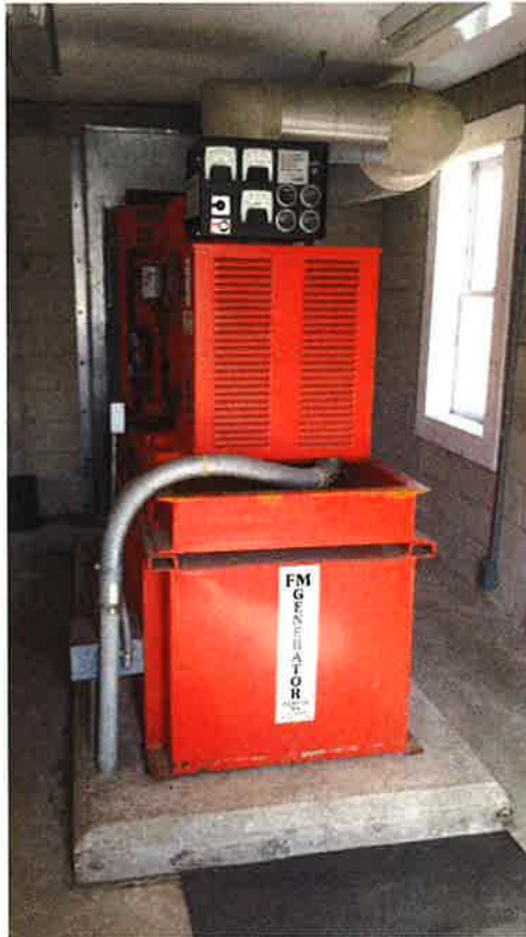
Figure 6: The existing emergency generator at the South Valley PS.
