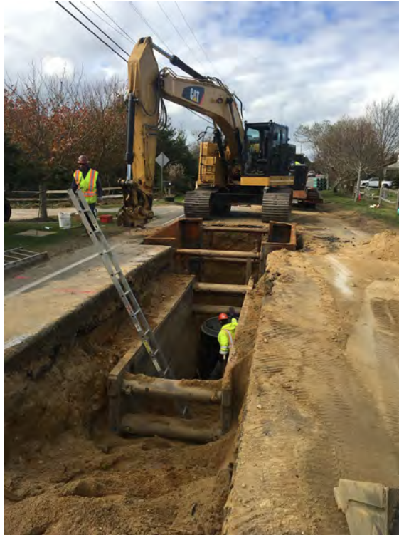
Wastewater (Sewer and Septic)
