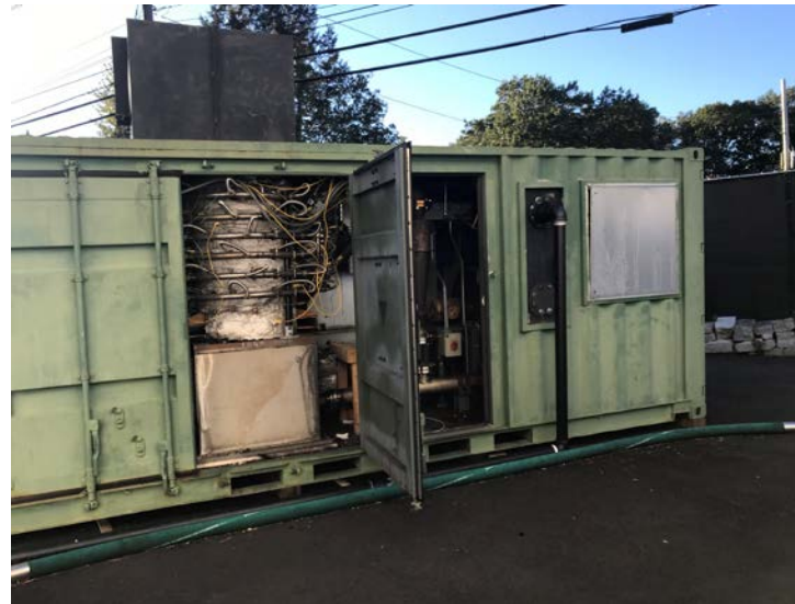
Containerized pyrolysis unit for plastics processing, Concord, Mass.
