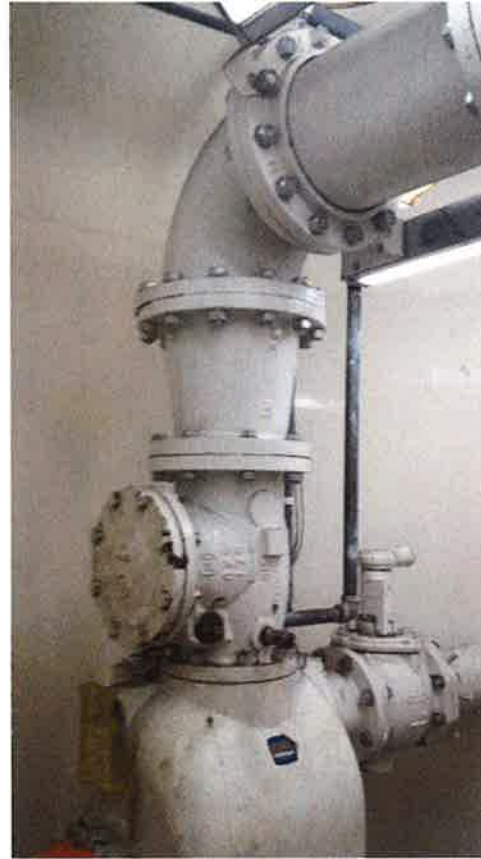
Figure 7: Gorman Rupp T6A3-B pump at South Valley PS.
