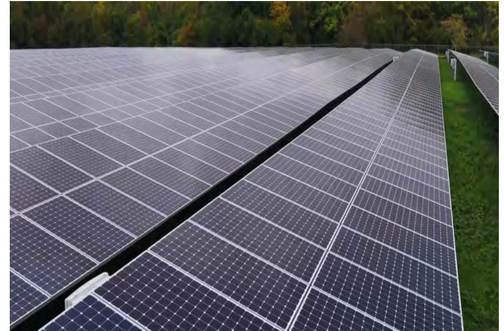
Photo of Campbell's Soup solar project installed by SunPower, similar in design to WWCo Wyers Valley Solar Project
