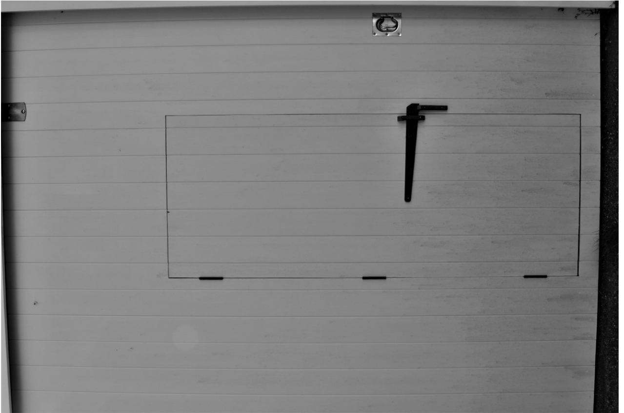
Photo #22 – Long Shed – north elevation - door cut into sliding door at 2 nd bay from east
