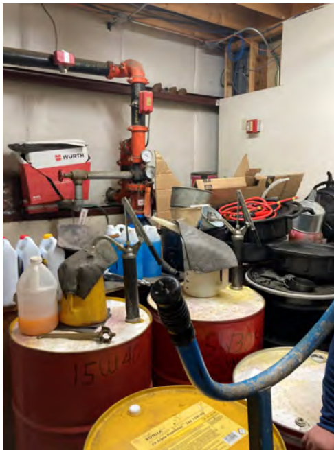
Fluid Storage Room
