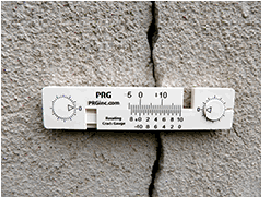
Concrete Crack Monitoring Gauge
