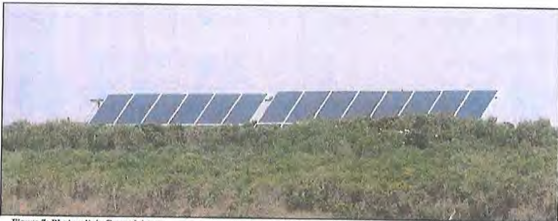
Figure 7: Photovoltaic Ground Array
