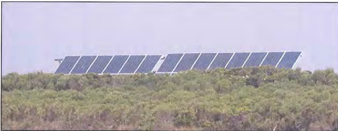
Figure 7: Photovoltaic Ground Array
