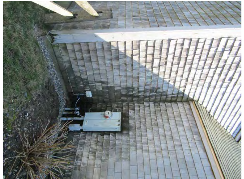
24. West elevation of main block (left) and north elevation of first ell (right) typical siding deterioration, view southeast
