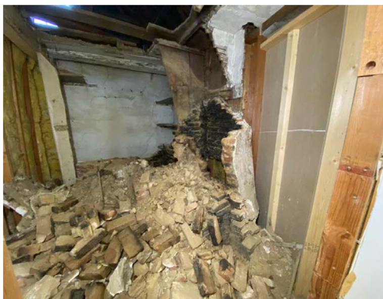
8. Second floor, collapsed former chimney stack, view west
