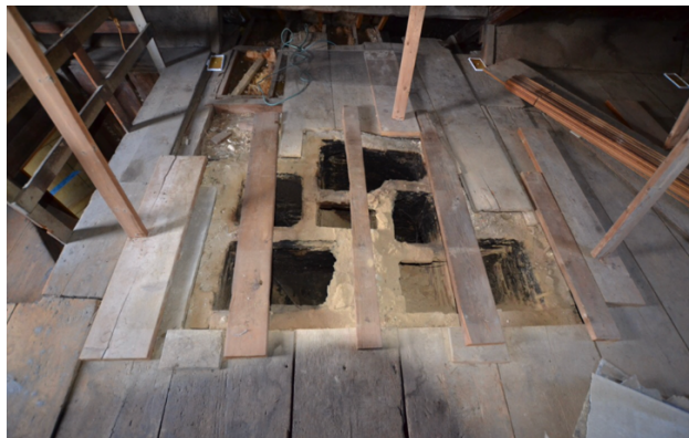
Exposed flues, documented under previous owner, 2019.
