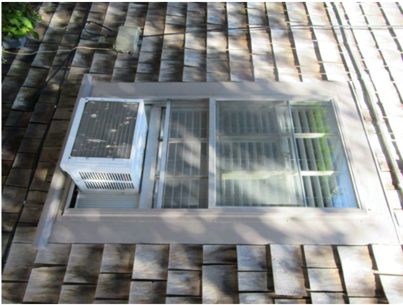
9. West elevation, window detail, typical conditions, view northeast
