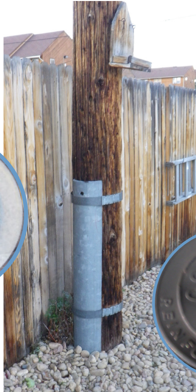
Installed in 1968 - In service 49 years and counting!
