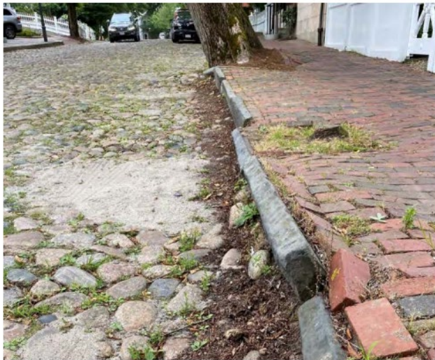
Shallow historic schist curb, likely unable to be re-used in this location.
