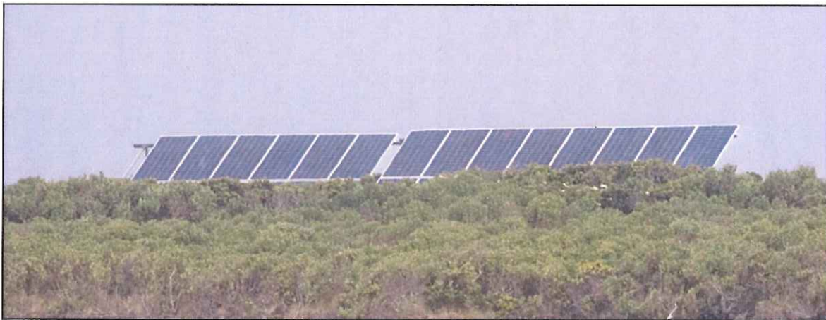
Figure 7: Photovoltaic Ground Array
